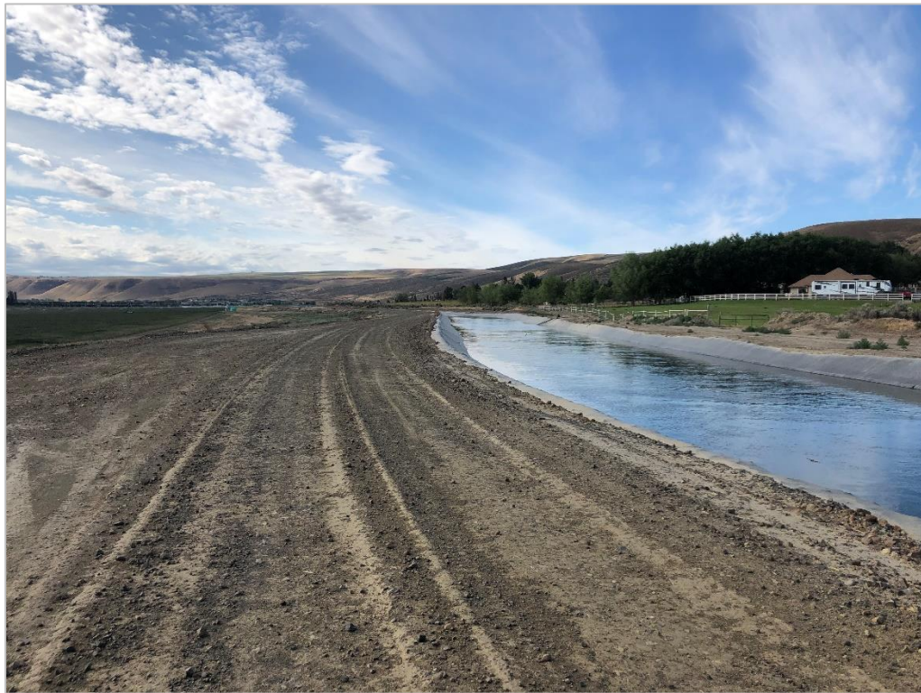
Figure 13. Overview of KID Main Canal Division III east of South Badger Canyon Road, Aspect: East
