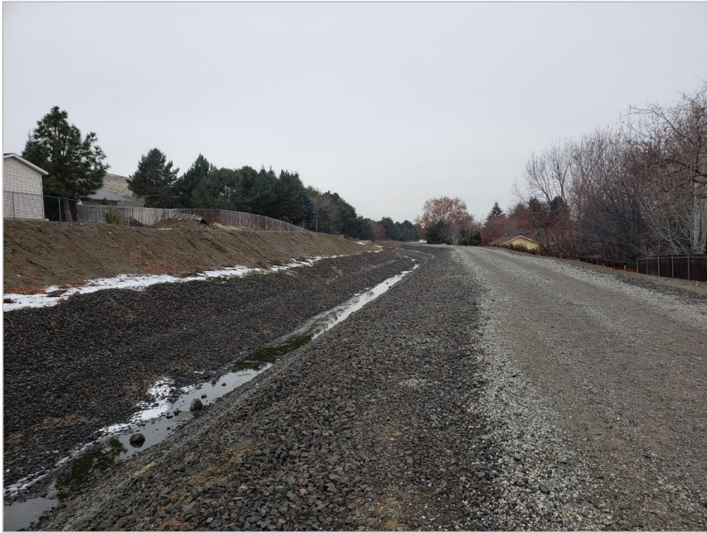
Figure 37. Overview of Highland Feeder Canal, West of South Columbia Center Blvd, Aspect: West
