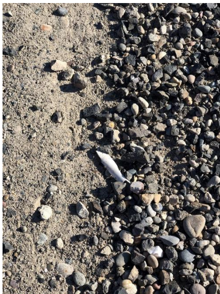
Figure 3. PVC Irrigation Pipe Debris on Badger East Lateral
