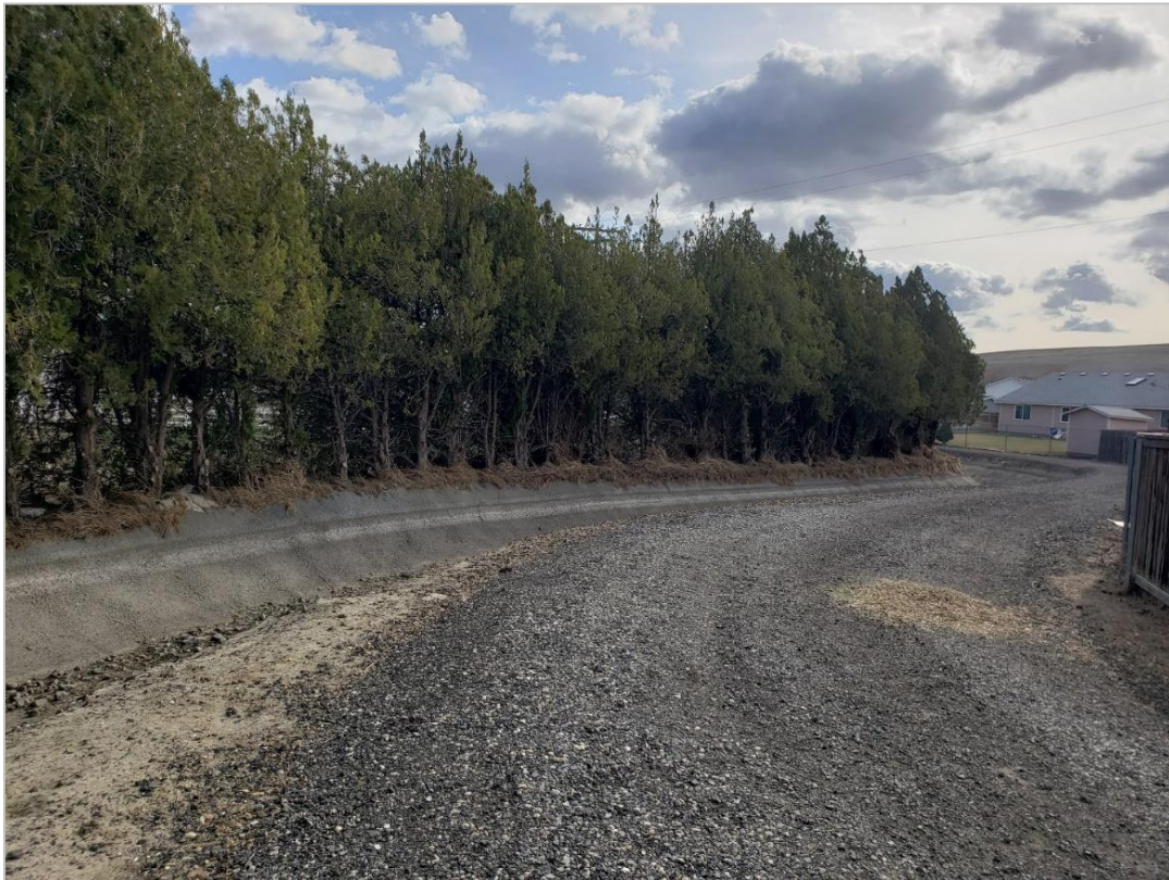
Figure 33. Overview of Highlift Canal, West End North of W 45th Ave, Aspect: Southeast
