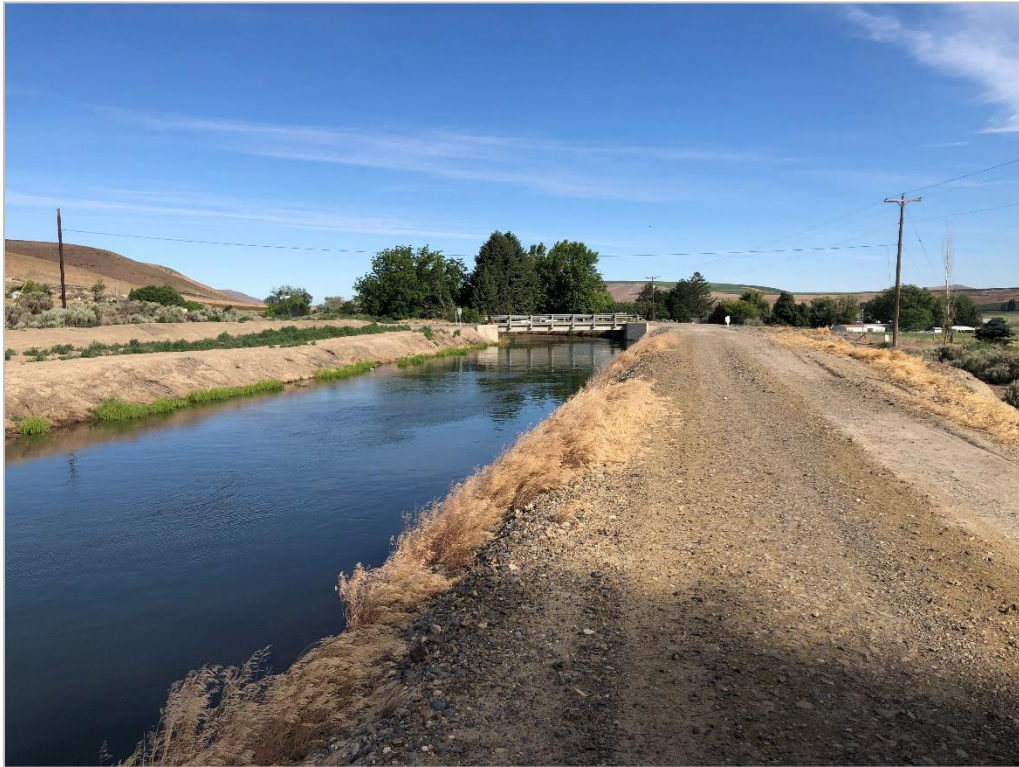
Figure 11. Overview of KID Main Canal Division III near N Bridge PR NE, Aspect: West
