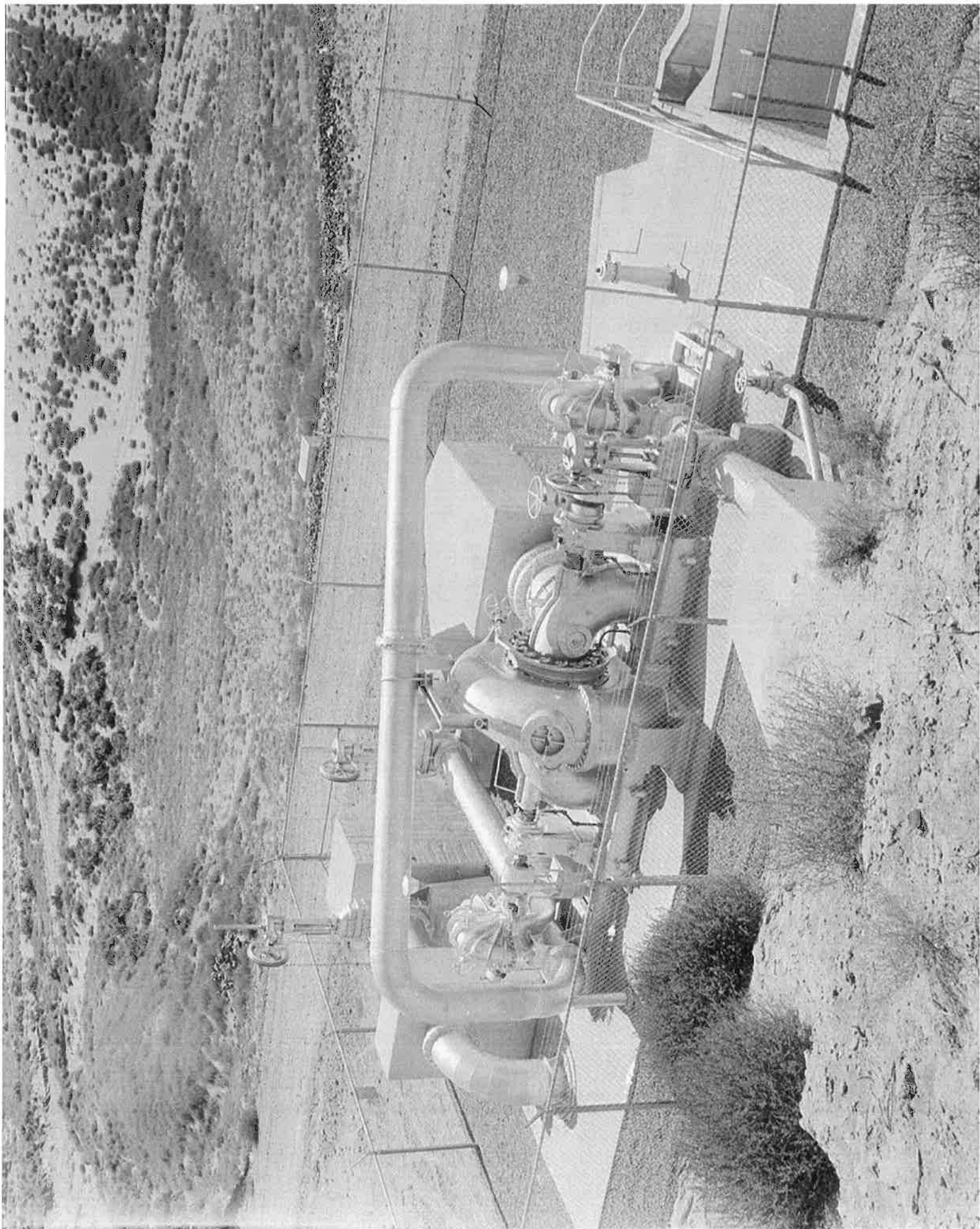
P566-121-1493 Kennewick Division View looking down on Amon Pumping Plant from siphon service road (Specifications DC-4323). Yakima Project, Washington. Photographer unknown. 7/18/1956.
